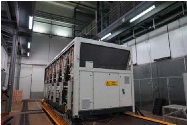
State of the art Large Air-Cooled Test Facility (LACTF) to test, qualify and optimize performances
